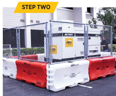
Fence and crash barrier
