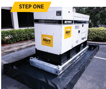
X-Guard containment berm
