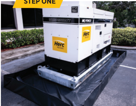
X-Guard containment berm
